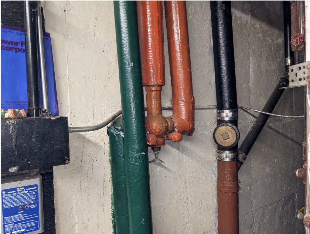
Photo #10: Typical Domestic Hot Water Mixing Valve
