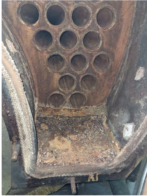
Photo #5: Boiler Tubes
