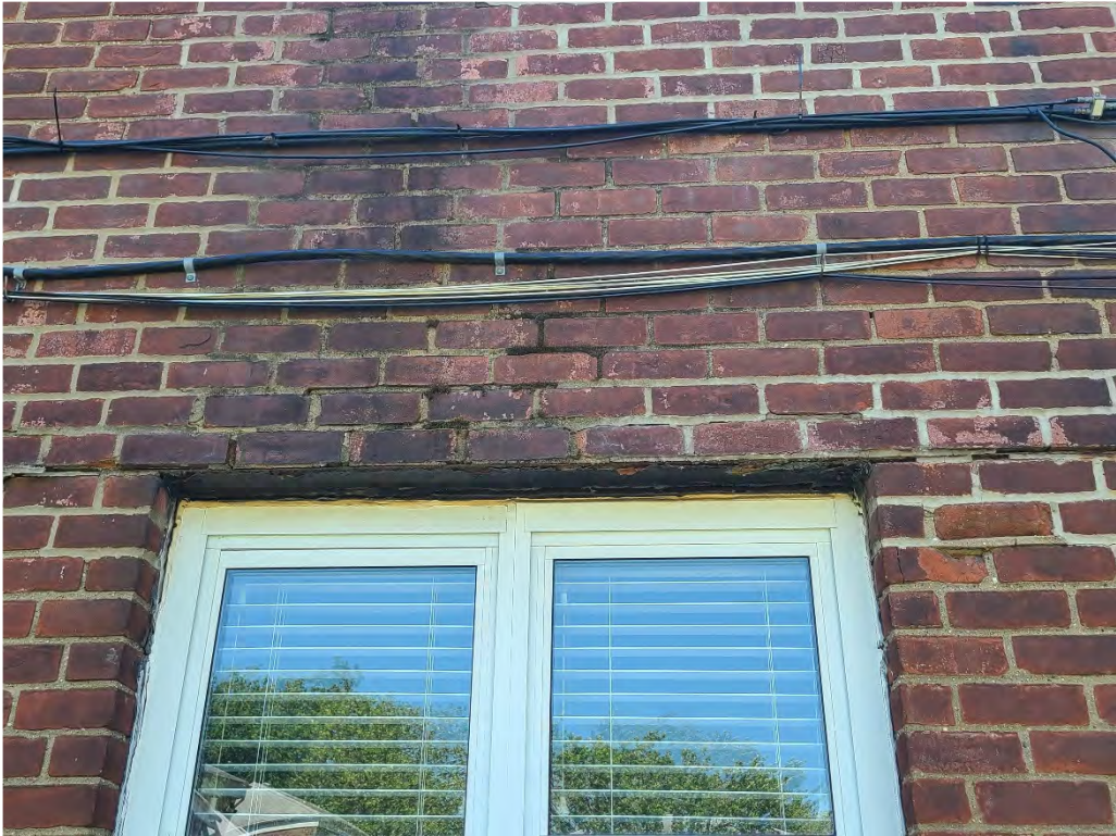
Photo # 12: Deteriorated lintel
