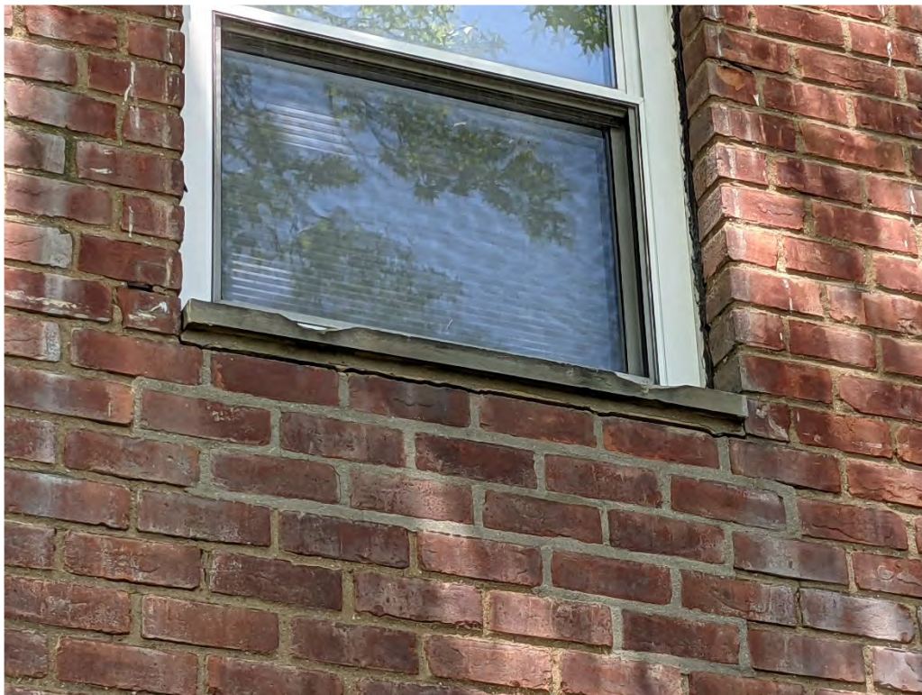
Photo # 2: Open joint at sill
