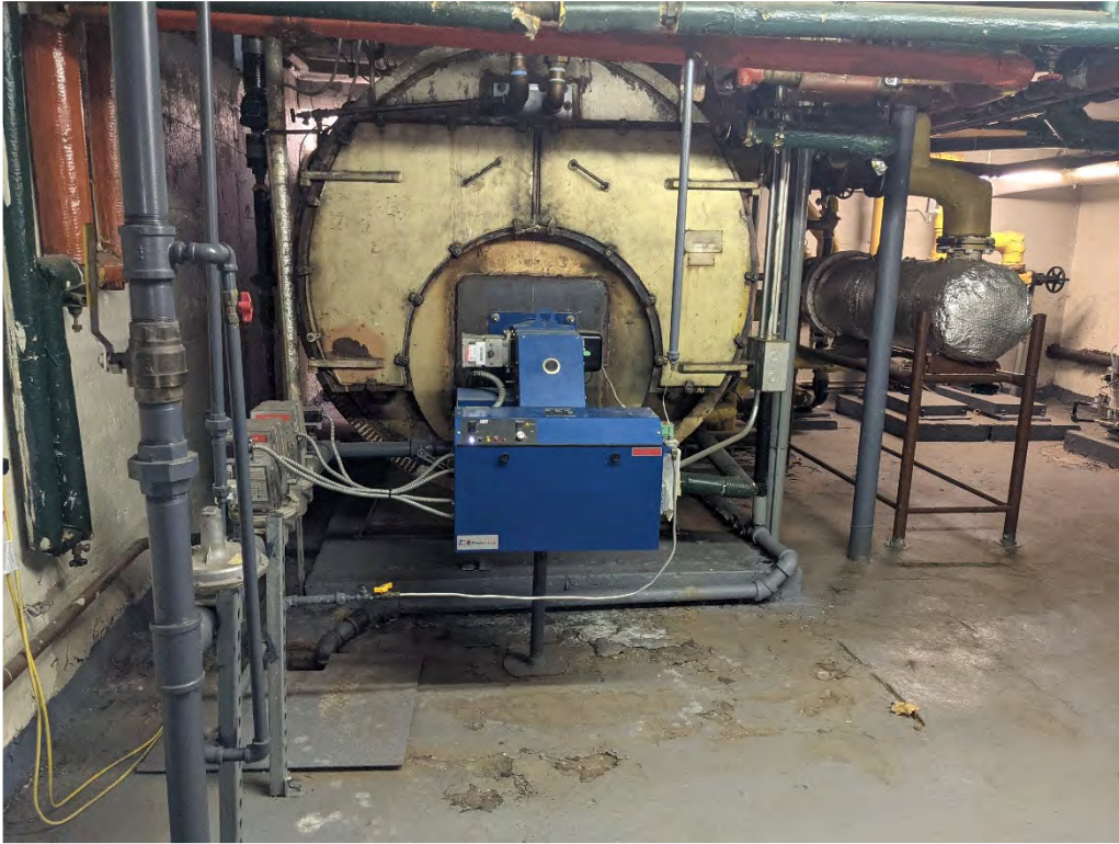
Photo #3: Typical Boiler, Burner, and Heat Exchanger
