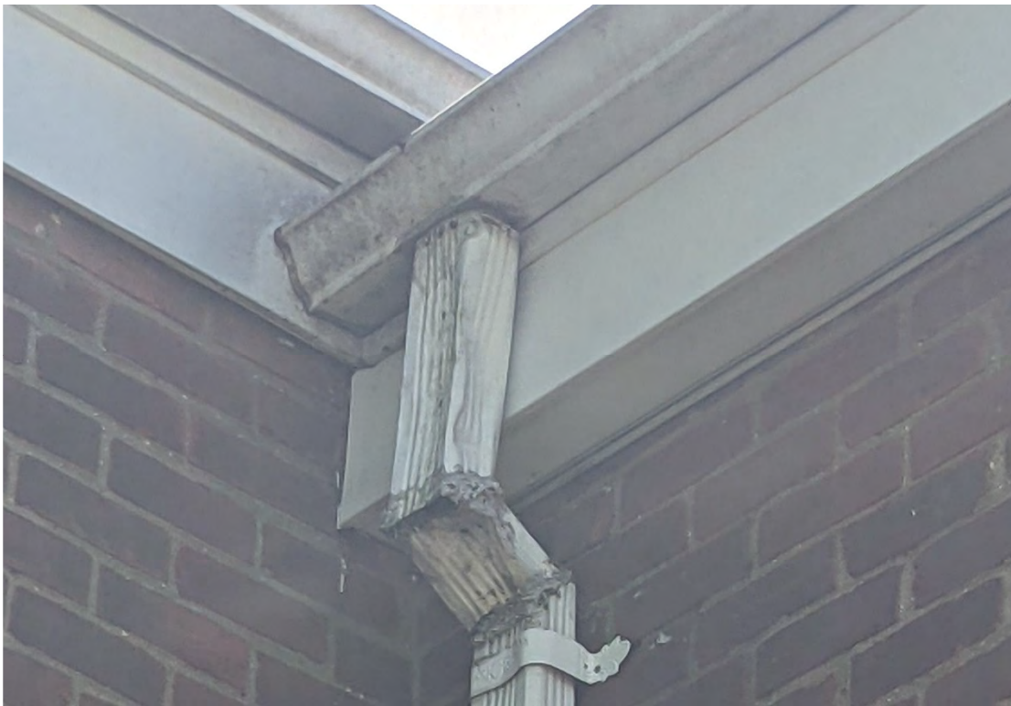
Photo # 4: deteriorated down spouts
