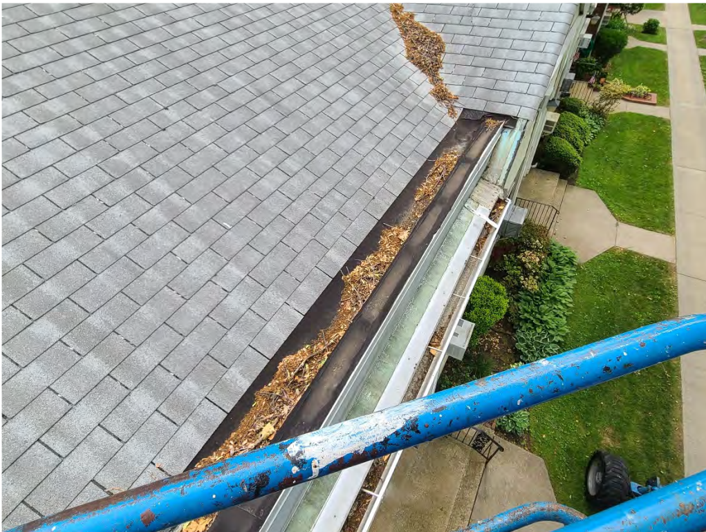
Photo # 2: Water run off diversion, debris, and aluminum gutter systems
