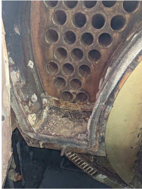
Photo #6: Boiler Tubes
