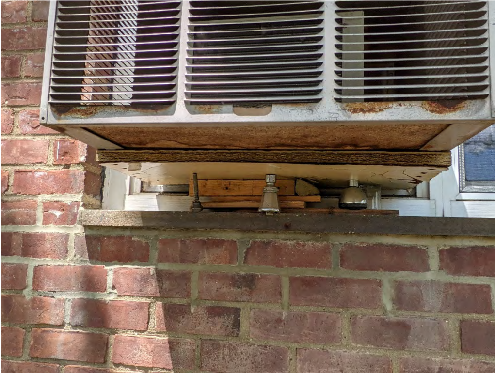
Photo # 7: improper window AC supports.
