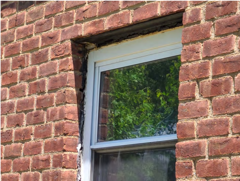
Photo # 4: Deteriorated window caulk
