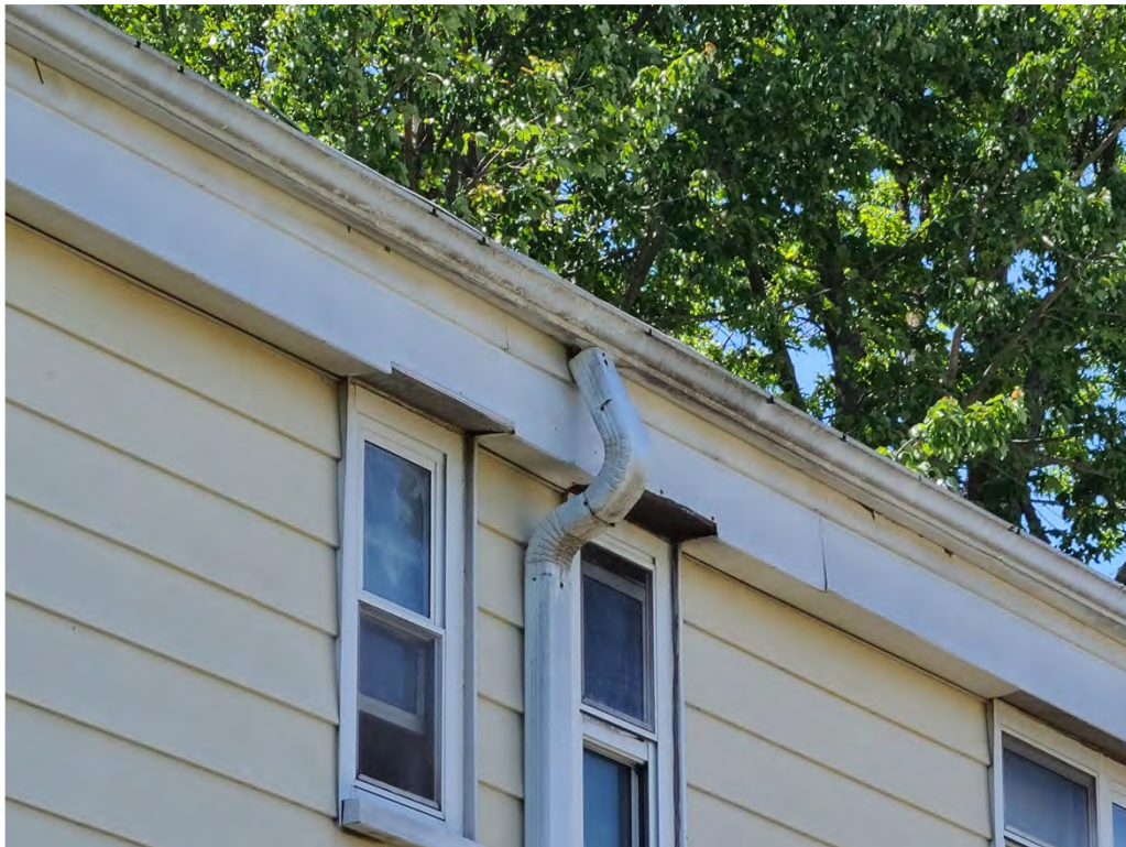
Photo # 8: Deteriorated gutters
