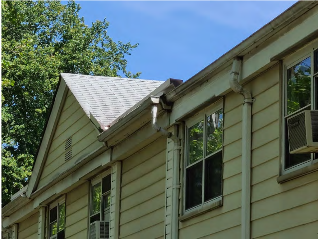
Photo # 7: Water diversion and gutter system
