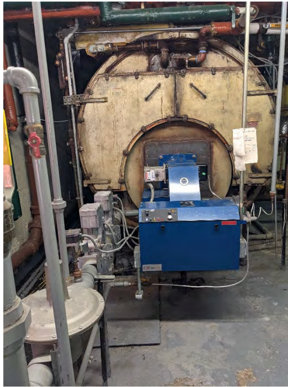
Photo #1: Typical Boiler and Burner
