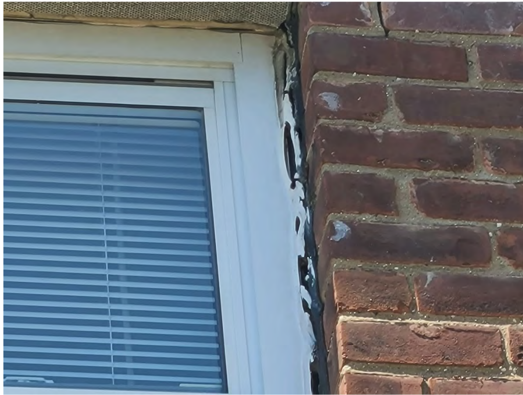
Photo # 5: Deteriorated window caulk
