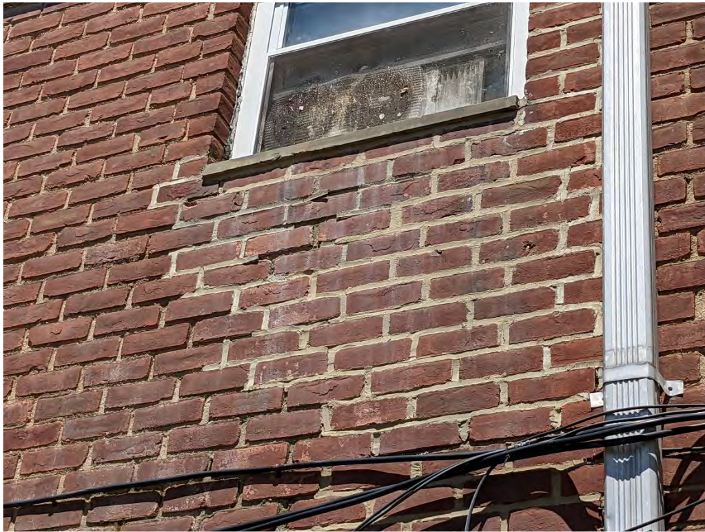
Photo # 1: Deteriorated mortar joints
