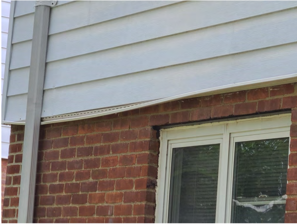
Photo # 9: loose siding trim
