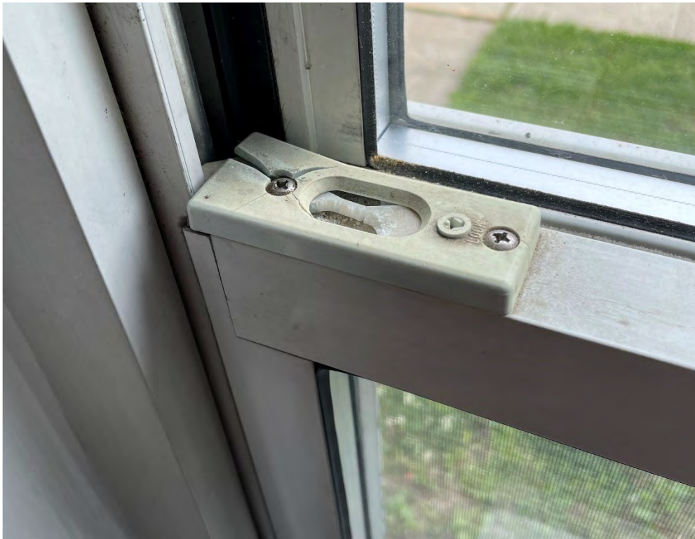
Photo # 2: Damaged tilt latch
