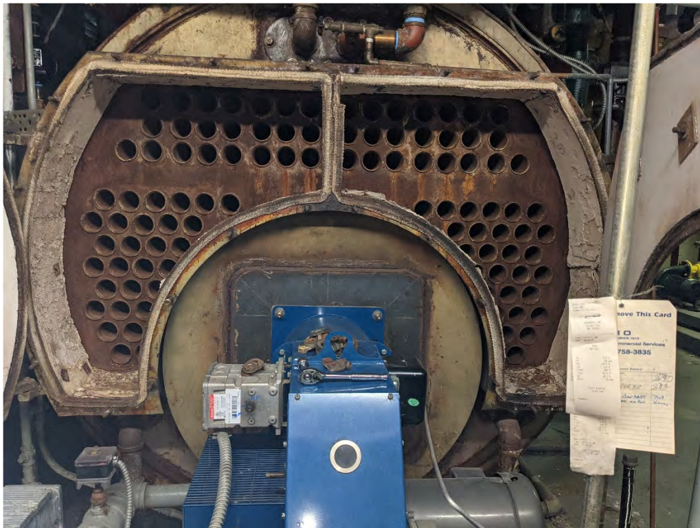
Photo #2: Typical Boiler with access door open
