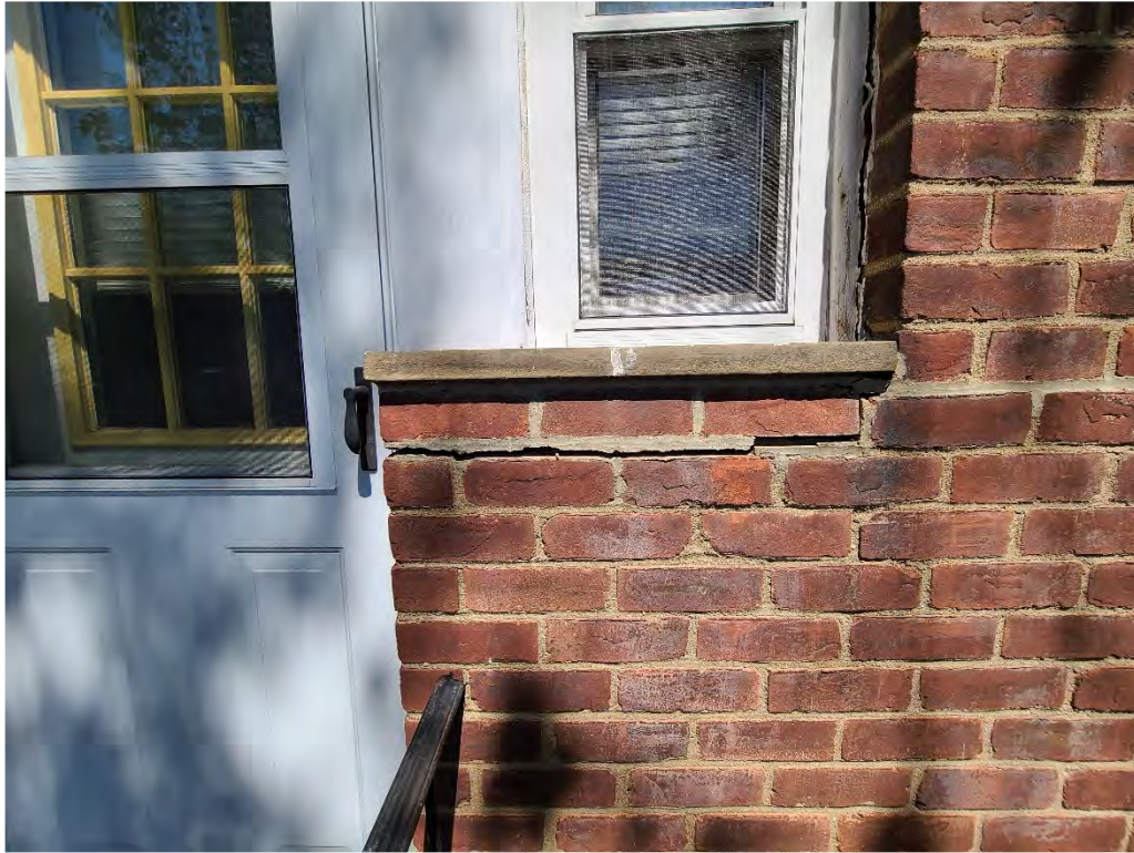
Photo # 5: Open mortar joints
