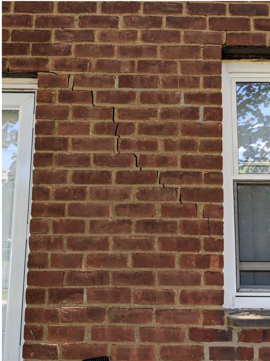
Photo # 3: Open mortar joints and cracked brick
