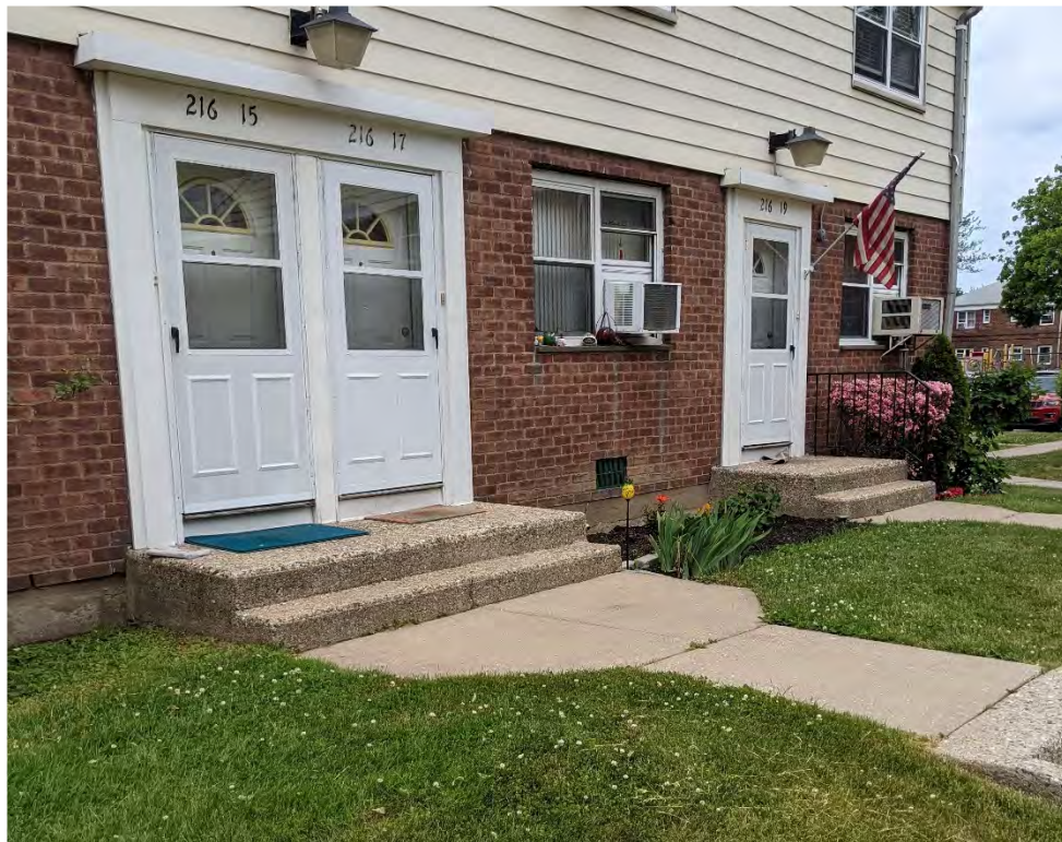
Photo # 6: missing handrails - Bldg. 32
