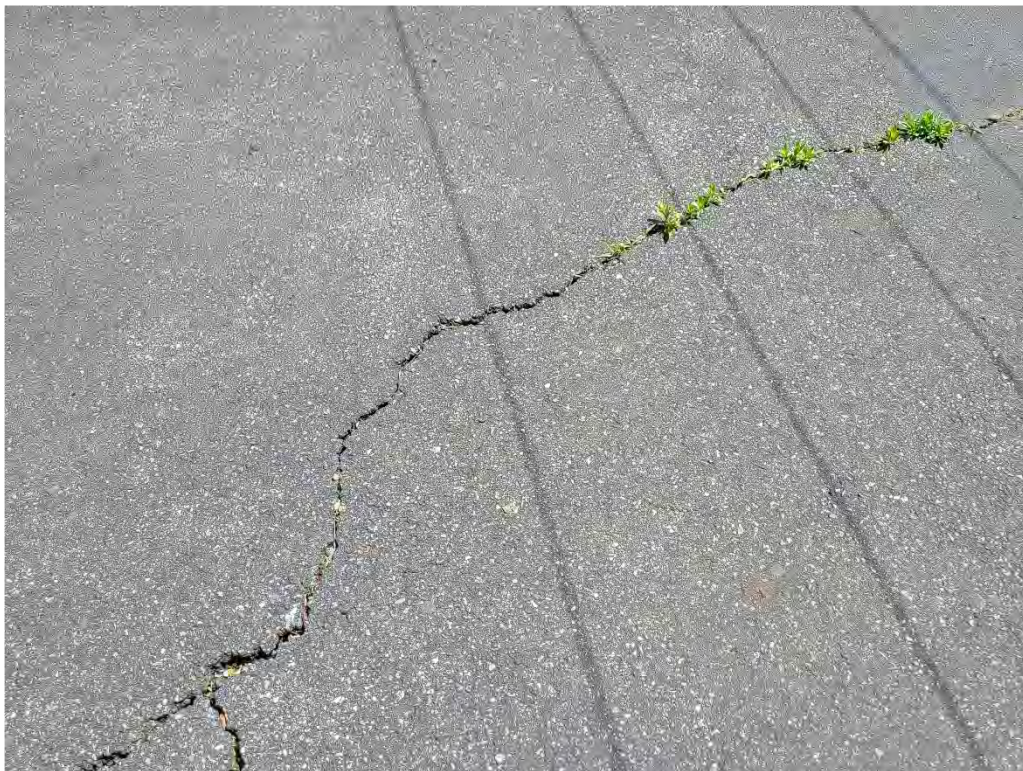
Photo # 2: Crack at asphalt – Bldg. 32
