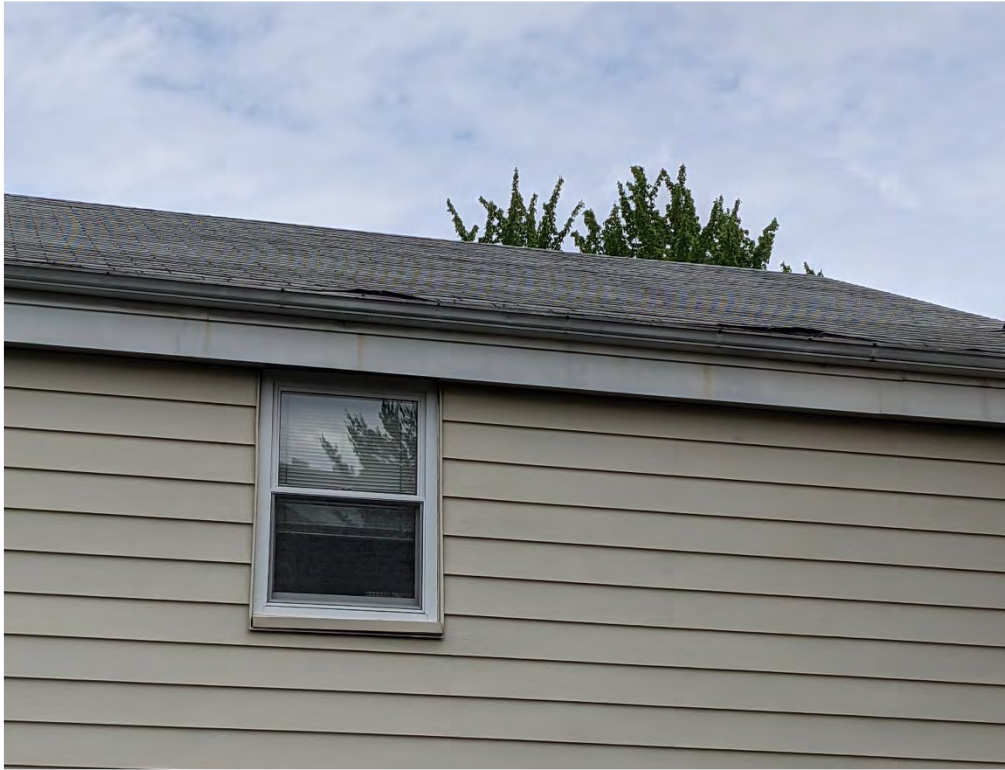
Photo # 3: Deteriorated roofing
