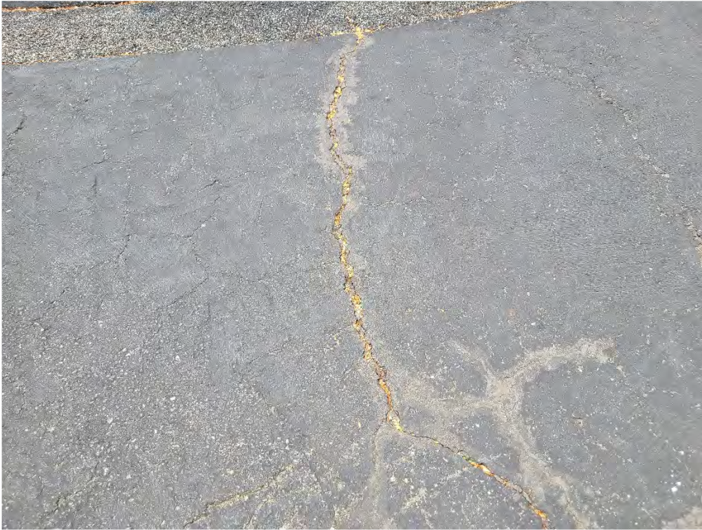
Photo # 3: Crack at asphalt - Bldg. 13
