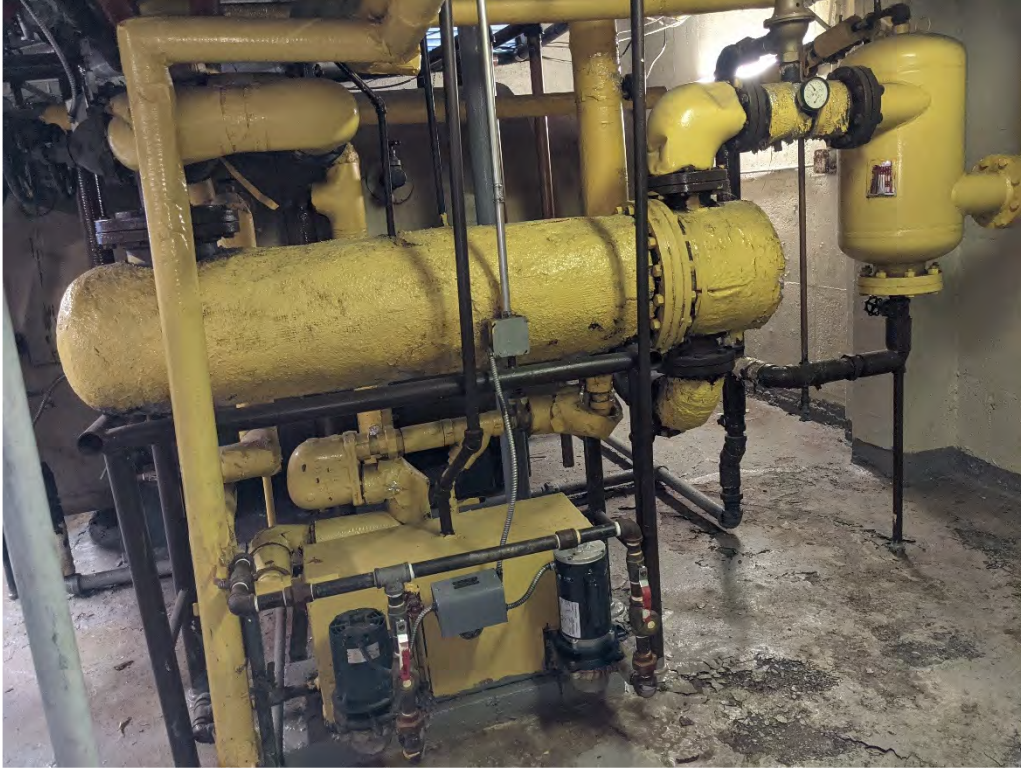
Photo #8: Typical Steam to Hot Water Heat Exchanger, Condensate Pump & Air Separator
