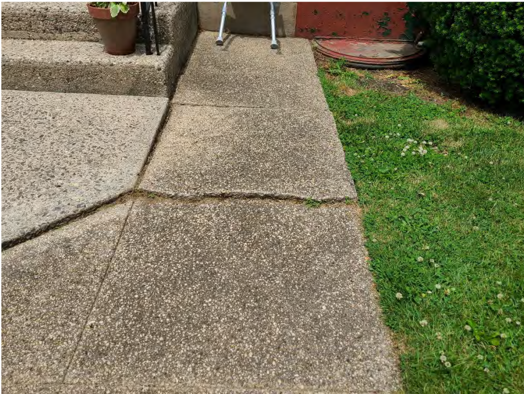
Photo # 4: Cracked/Heaved concrete flag - Bldg. 39
