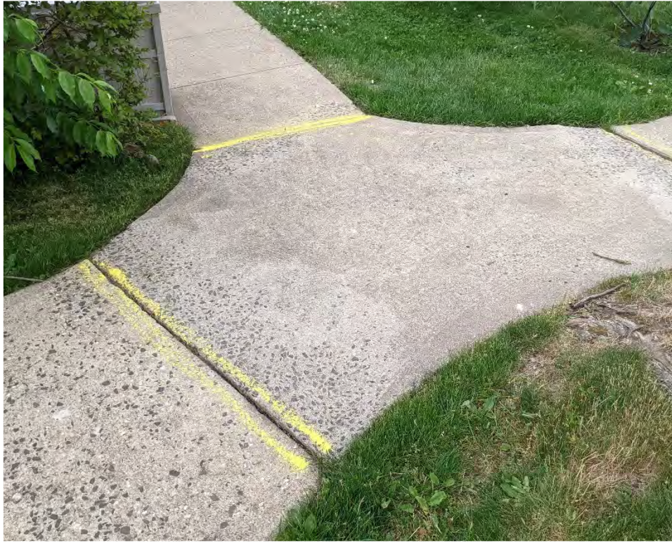
Photo # 7: heaved concrete flag - Bldg. 24
