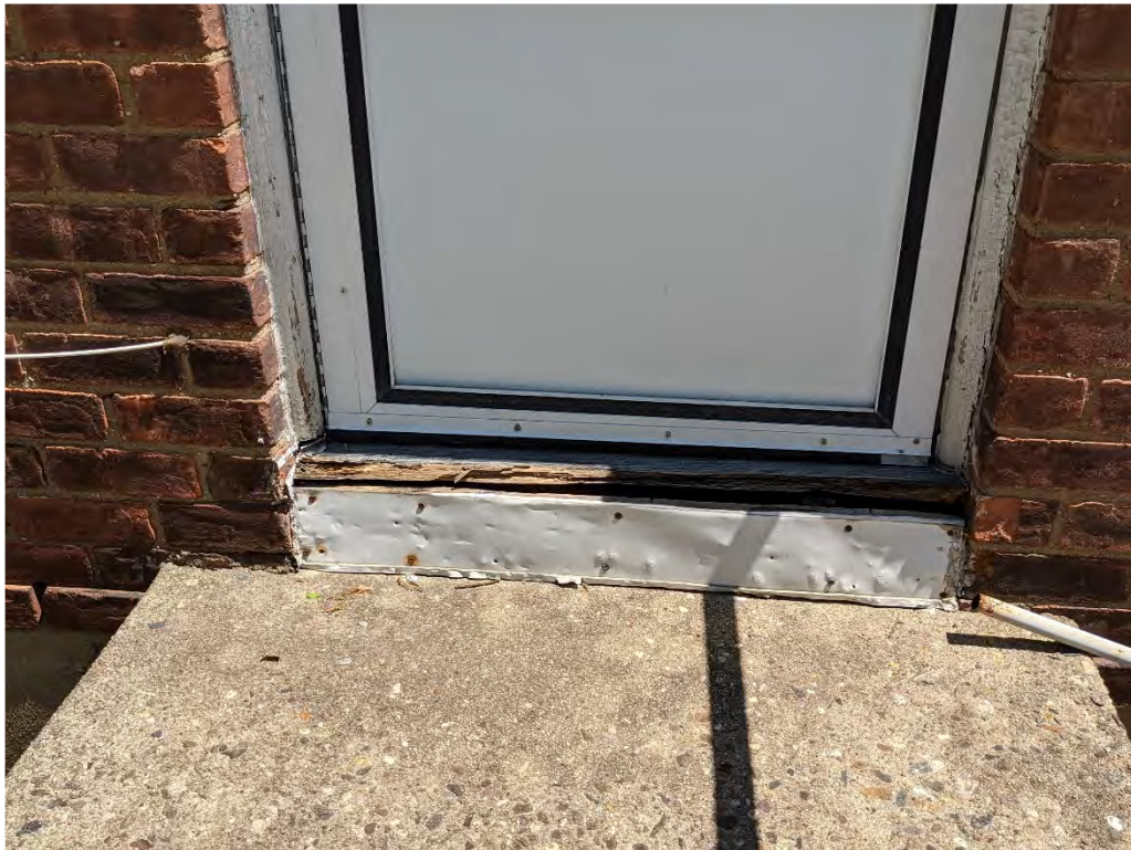
Photo # 6: Deteriorated wood stool
