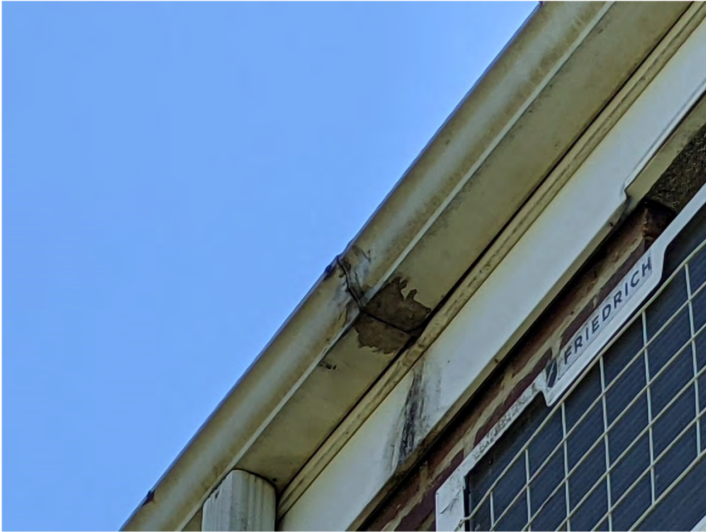
Photo # 5: Deteriorated gutters
