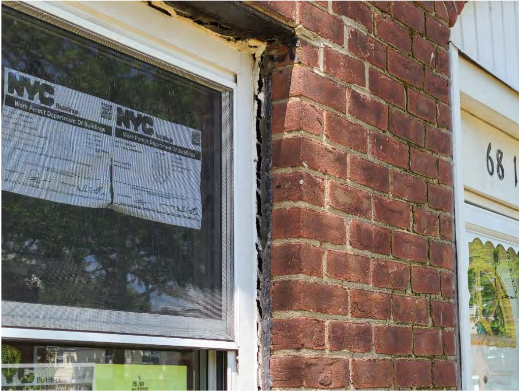
Photo # 3: Deteriorated window caulk
