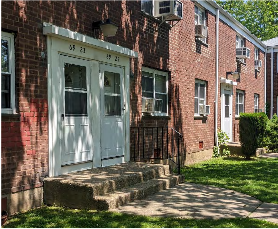
Photo # 5: missing hand rail - Bldg. 21
