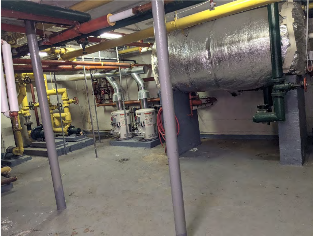
Photo #9: Typical Domestic Hot Water Storage Tank
