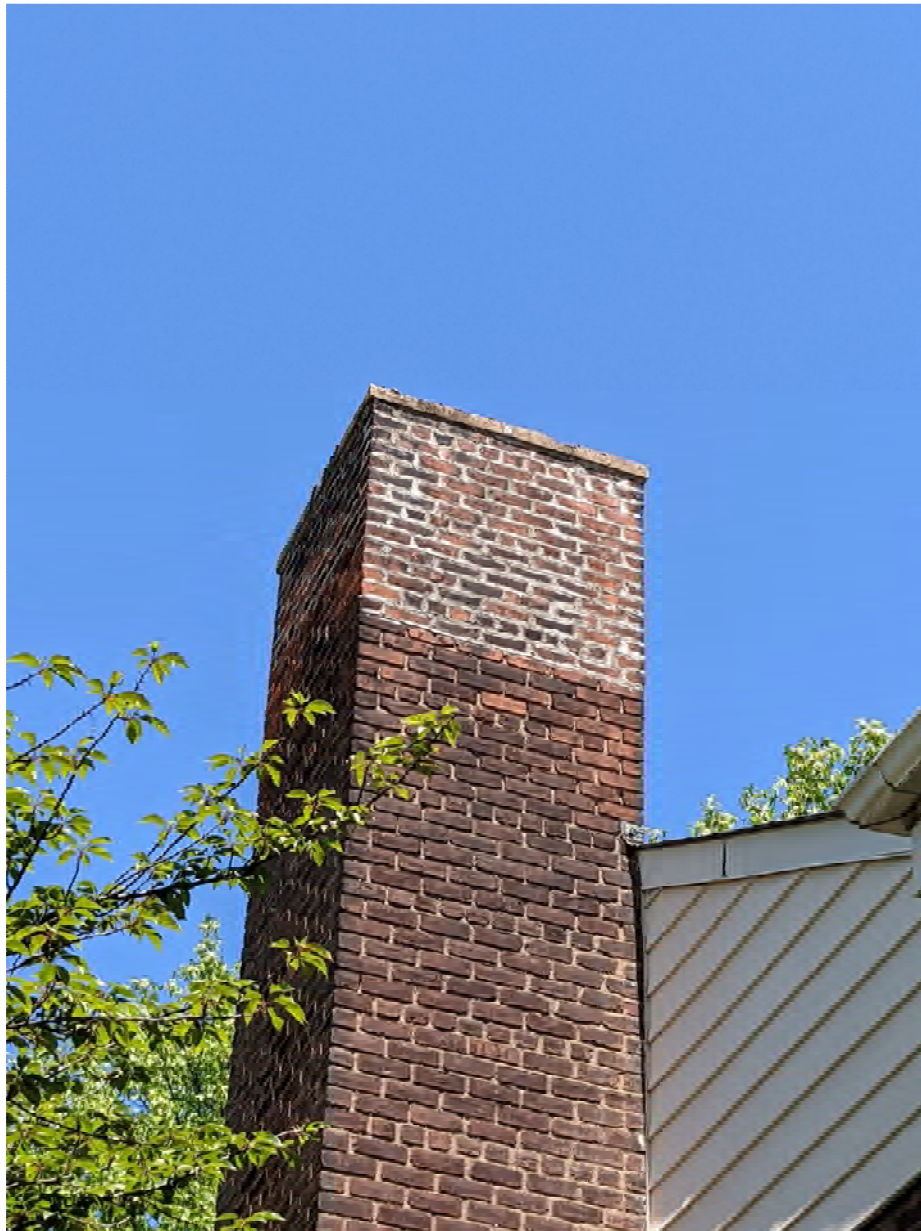
Photo # 4: Deteriorated mortar joints at chimney
