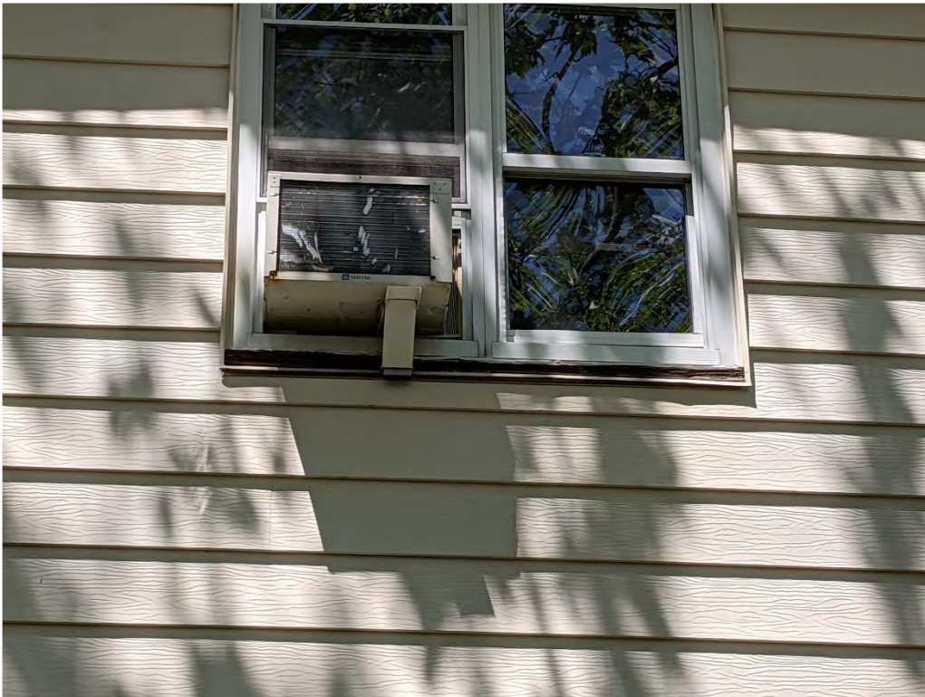
Photo # 8: Deteriorated window sill at siding
