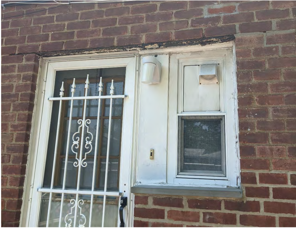
Photo # 11: Deteriorated lintel
