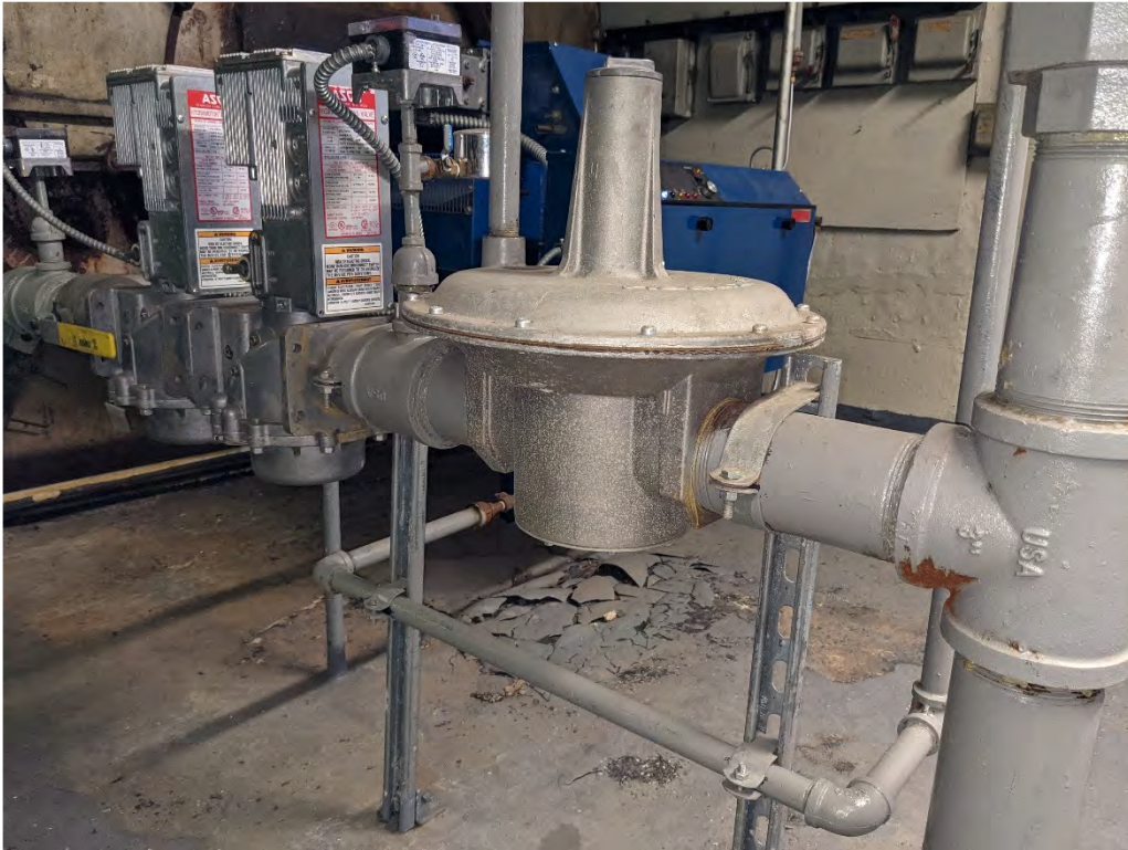
Photo #12: Typical Boiler Gas Train
