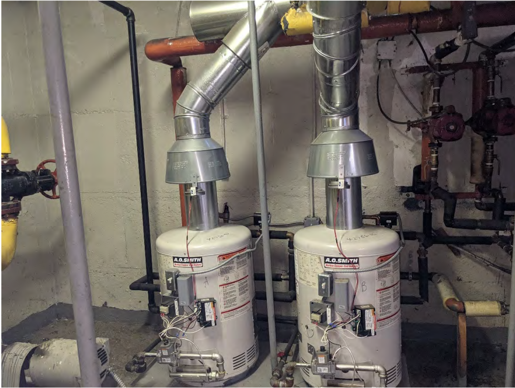
Photo #11: Typical Domestic Water Heaters
