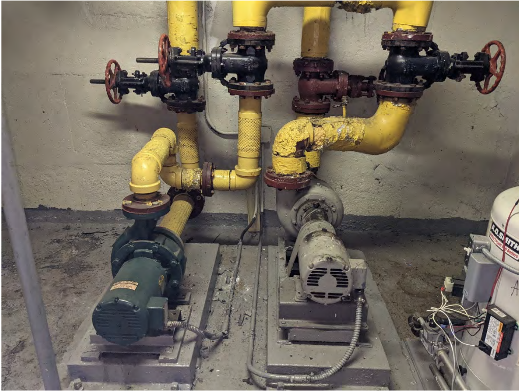
Photo #7: Typical Heating Hot Water Circulation Pumps (Replaced Pump & Original Pump)
