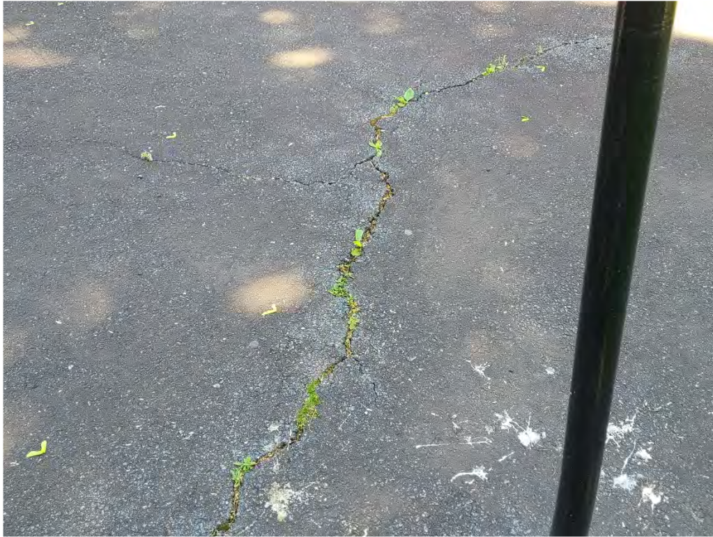
Photo # 1: Crack at asphalt - Bldg. 24
