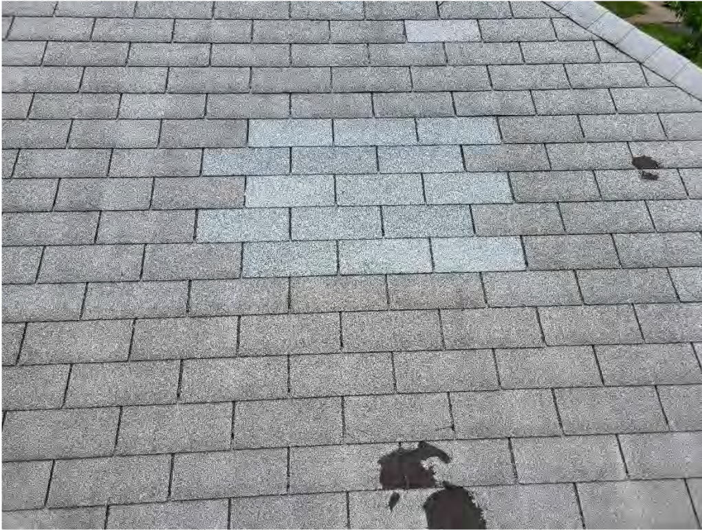
Photo # 1: Roof patches - typical
