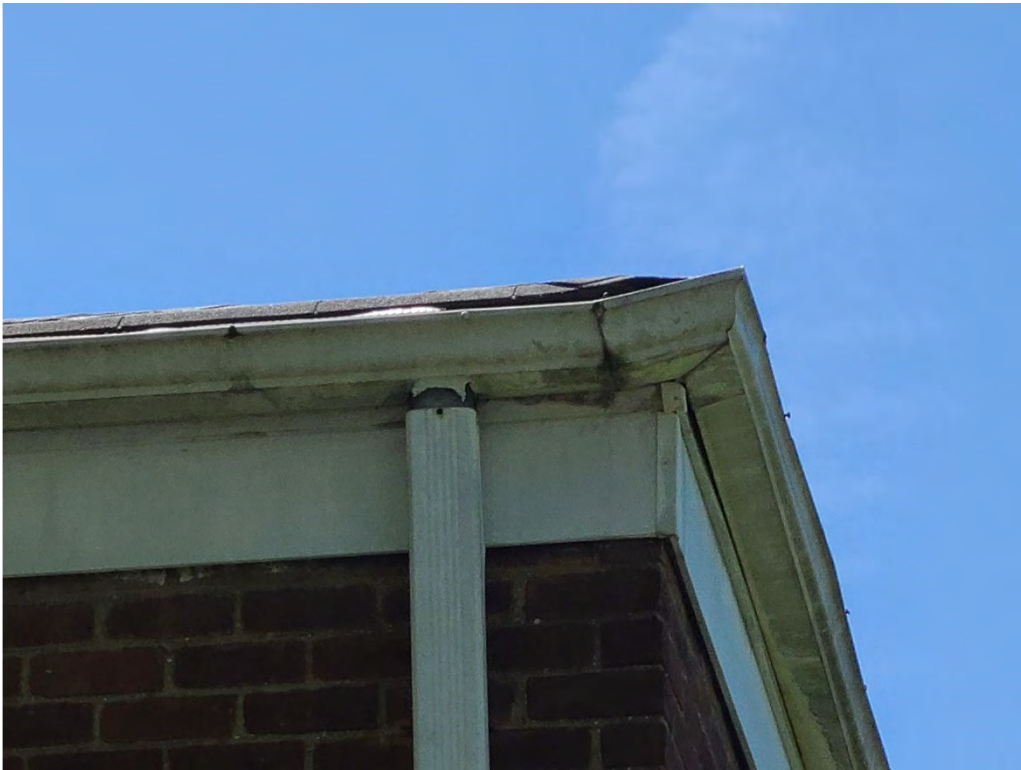
Photo # 6: Deteriorated gutters
