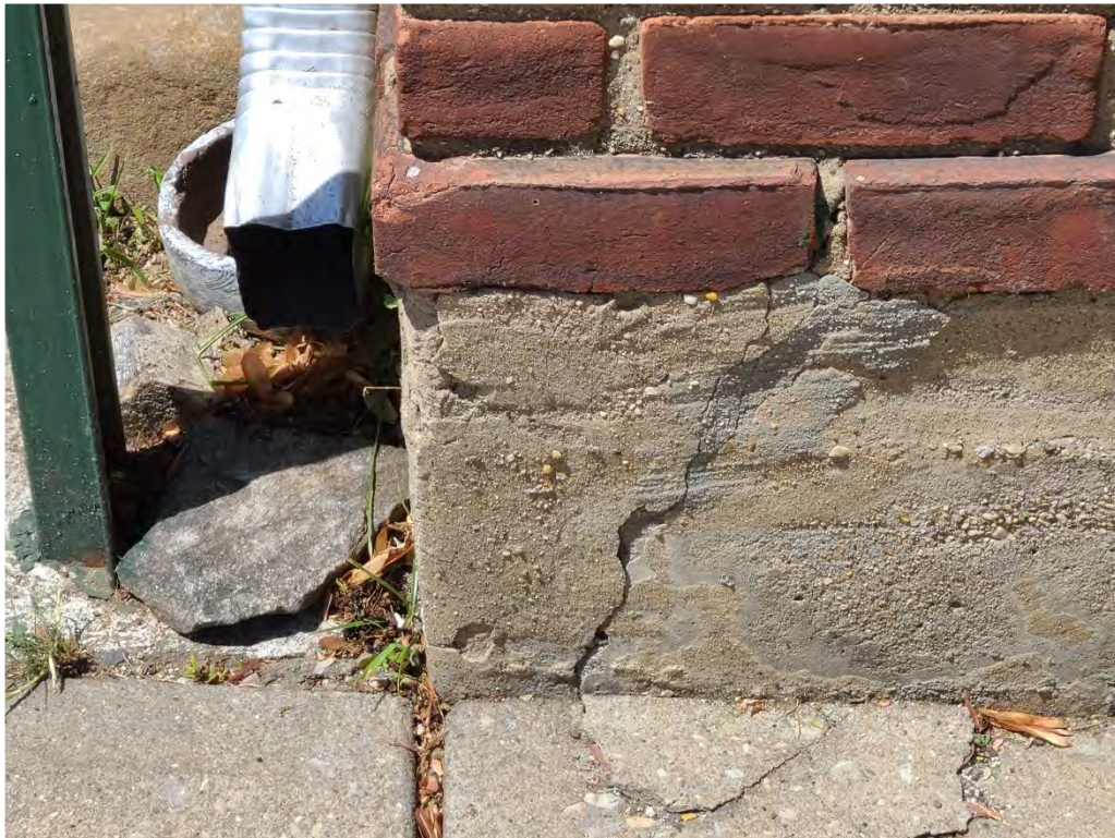
Photo # 10: Deterioration at foundation/stucco finish
